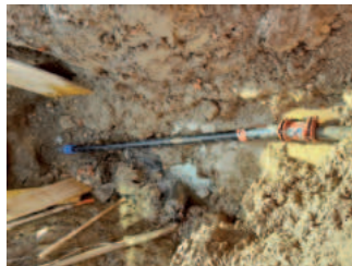
Wasserrohrbruch in Trautenfels
